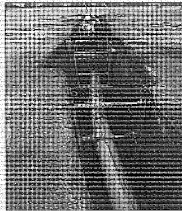
Pipe Bend on Ice Drive
