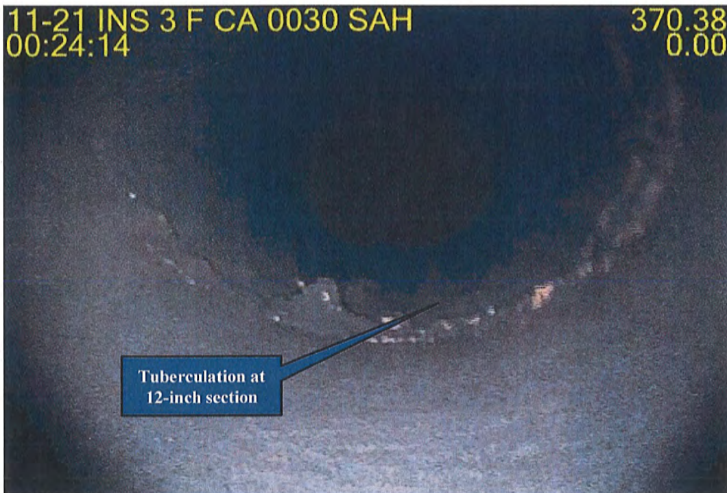
Figure 3.10: Tuberculation throughout 12-inch Steel Section
