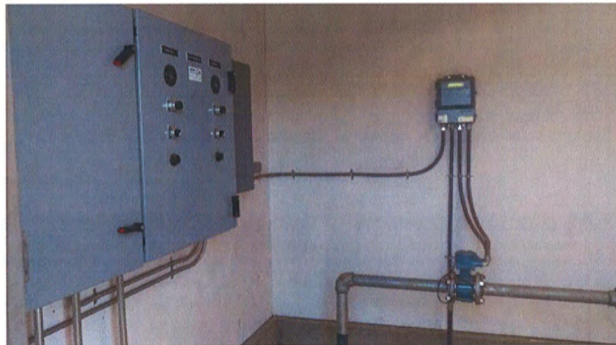
Windhaven Pump Station Interior (8/20/2015) (See Photo Location # 9 on Slide 2)
