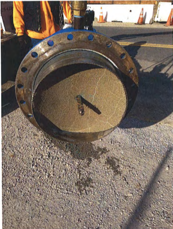
11/12/2013 View of the Interior Coupon of the 30" Existing Pipe that was Cut Out for One of the Line Stops
