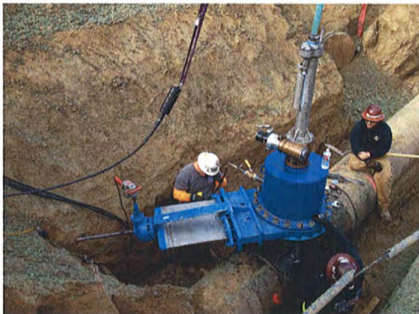
11/11/2013 Installing the Temporary Knife Gate and Hot Tap Machine at One of the Line Stops
