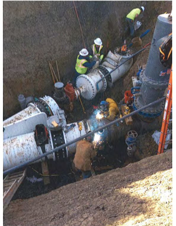
1/8/2014 Setting the Cut-In Pipe Spool at the North End Connection for W-1 Pipeline Segment
