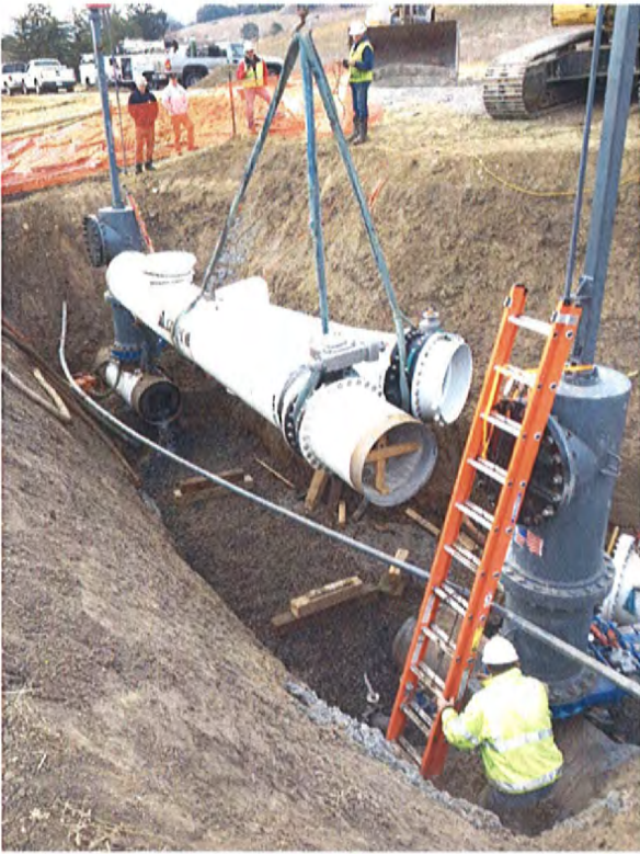
1/8/2014 Setting the Cut-In Pipe Spool at the South End Connection for W-1 Pipeline Segment
