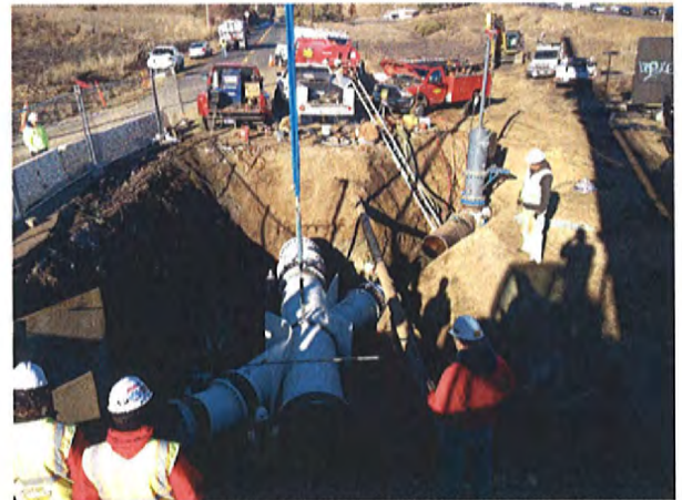
12/10/2013 Setting the Cut-In Pipe Spool at the North End Connection for W-2 Pipeline Segment
