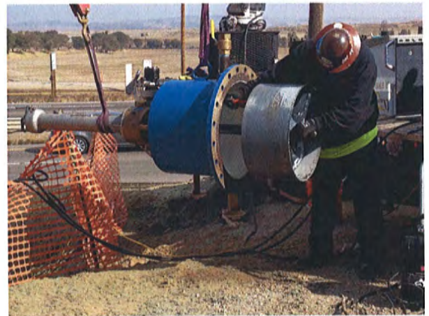
11/11/2013 Removing the Coupon from Hot Tap Machine at One of the Line Stop Locations
