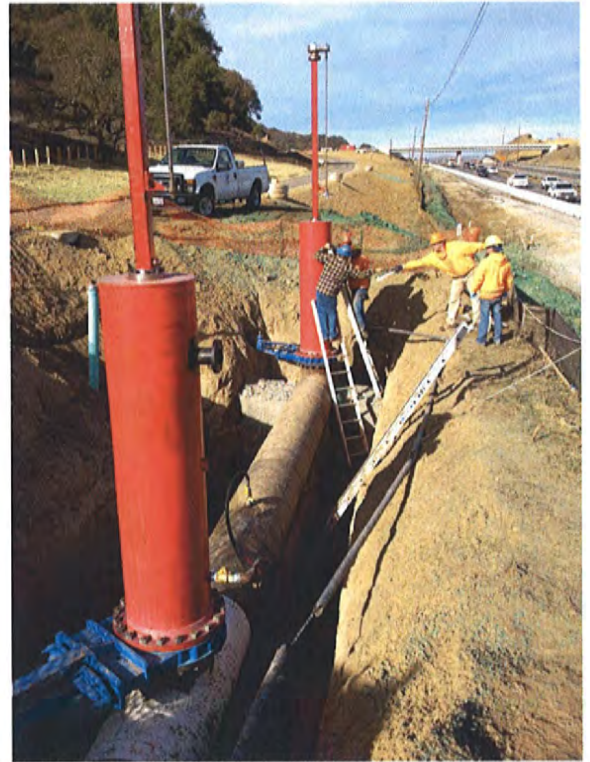
12/6/2013 View of Two Installed Line Stops at the South End of the W-2 Pipeline Segment
