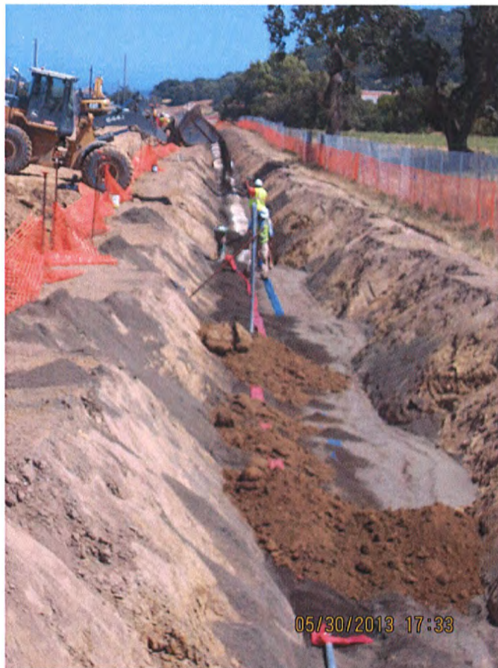
Installing the 2" PVC Telemetry Conduit on Top of the Pipe Zone Along with the Warning/ID Caution Tape
