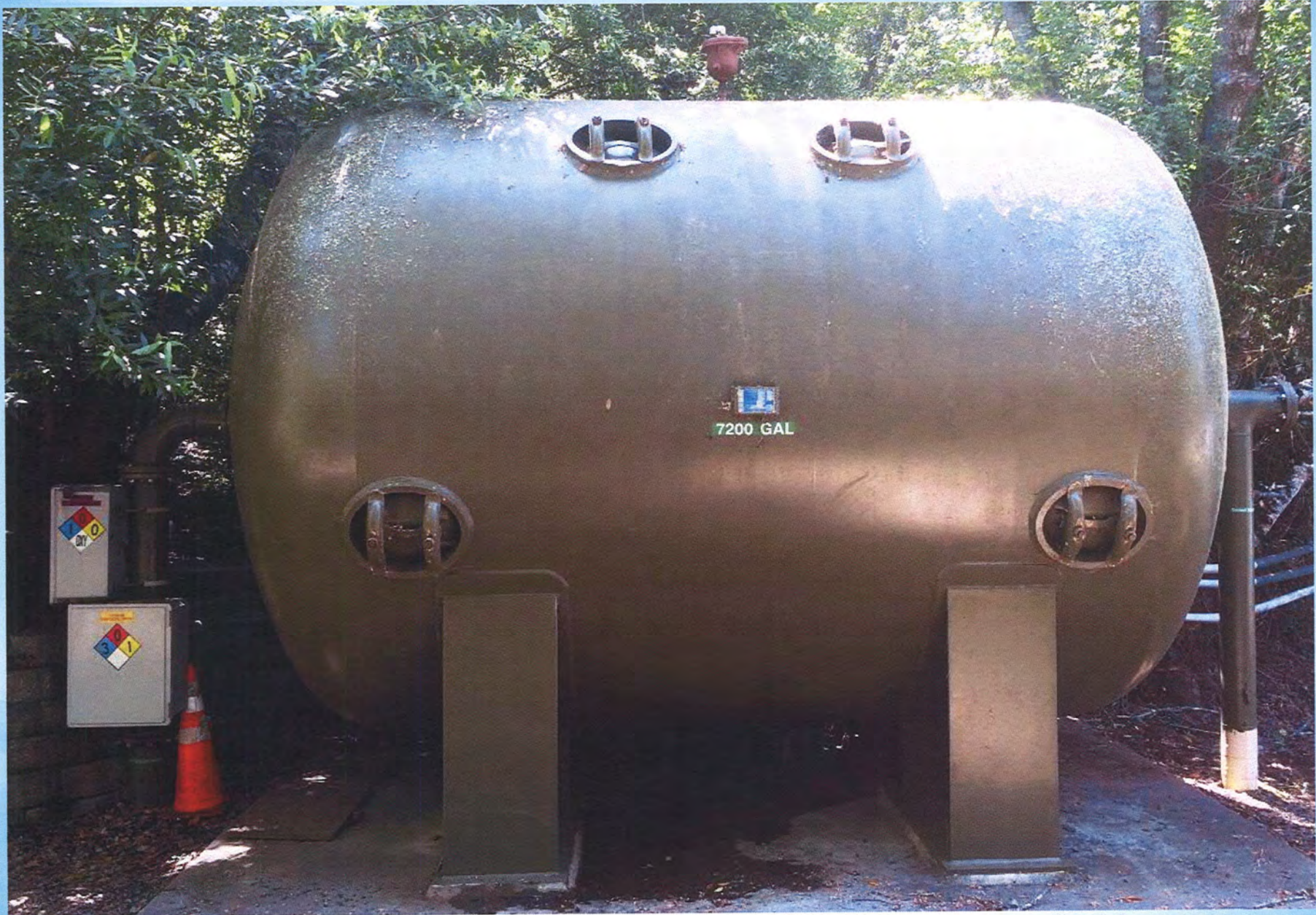
Chemical Contact Tank
