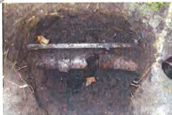
Photo showing broken sewer pipe- Google image courtesy of Rick Adams
