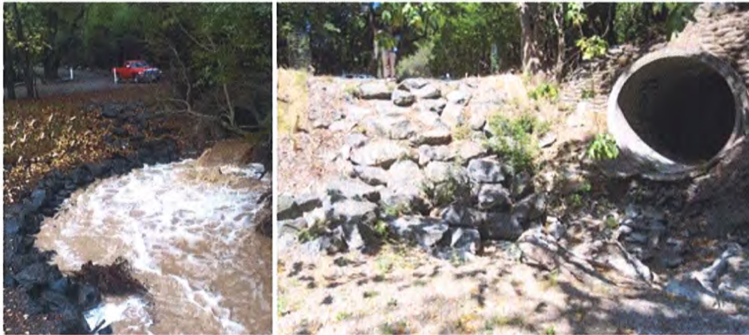
Figure 4. Culvert and downstream bank repair area during high flow (left) and after first year of high flows (right), looking upstream. Photos by NMWD (December 2012) and PCI (June 2013).
