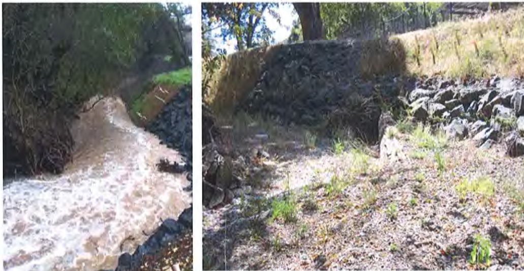
Figure 3. Project site during high flow (left) and in summer dry conditions after the first year of high flows looking downstream from culvert. Note that the rock and biotechnical treatments have remained stable. Photos by NMWD (December 2012) and PCI (June 2013).
