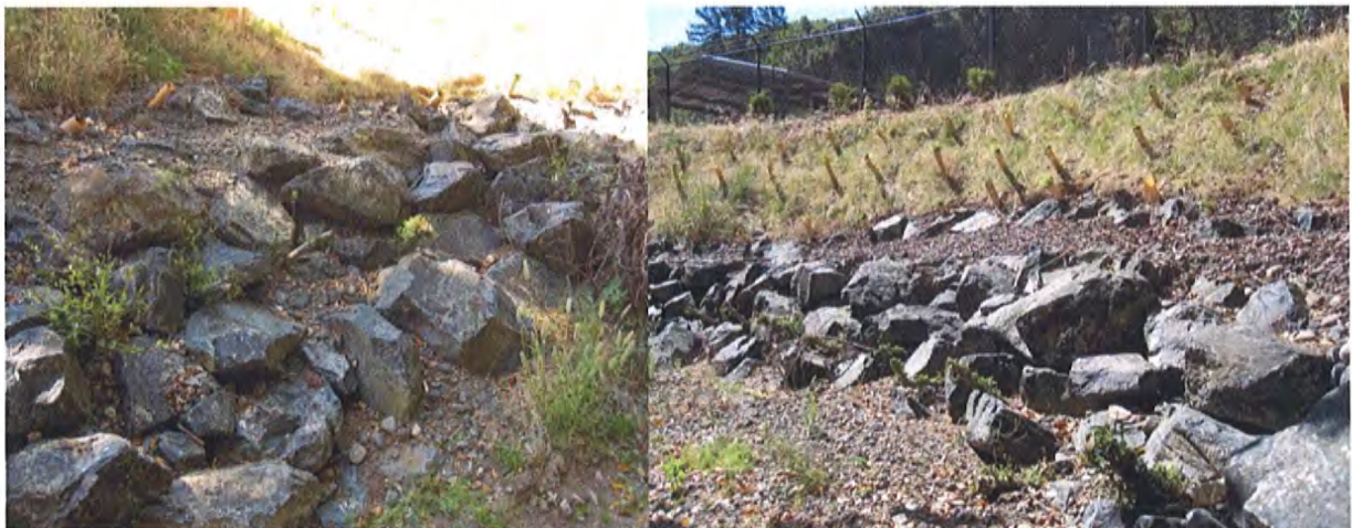
Figure 7. Photos showing willow and grass survival along the streambank repair (PCI 2013)
