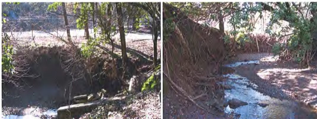
Figure 2. Pre-project bank erosion downstream of culvert. Photo on left looking across channel at erosion of concern, fence and road. Photo on right looking up channel at eroding bank.
