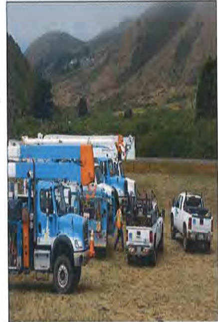
Pacific Gas & Electric Co. trucks and personnel gather in the Marin Headlands near Sausalito on Tuesday to upgrade transmission lines in the area.
