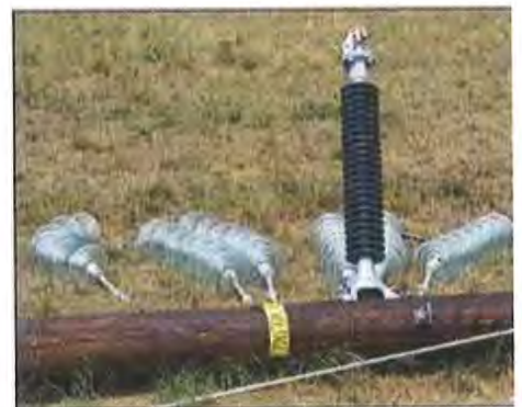
Pacific Gas & Electric Co. equipment sits in a staging area in the Marin Headlands.
