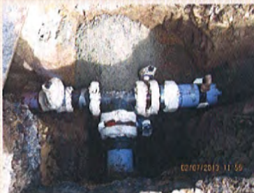
Hamilton Pkwy (J-Line) Tee and Valves
