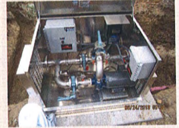
Irrigation Booster Pump at Hamilton School Site
