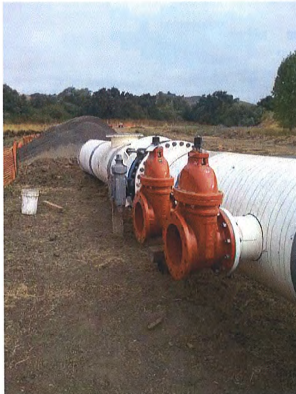
Connection for flexible hose by-pass system south of Creek (7)
