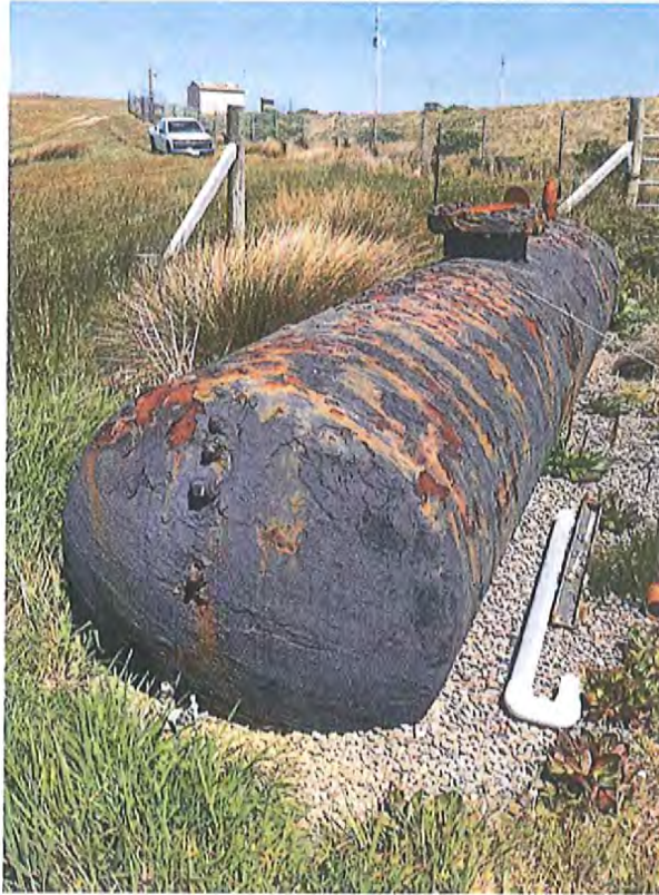
Oceana Marin Dosing Tank Before
