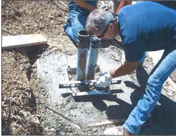
Bolling Circle RWF Pump Station
