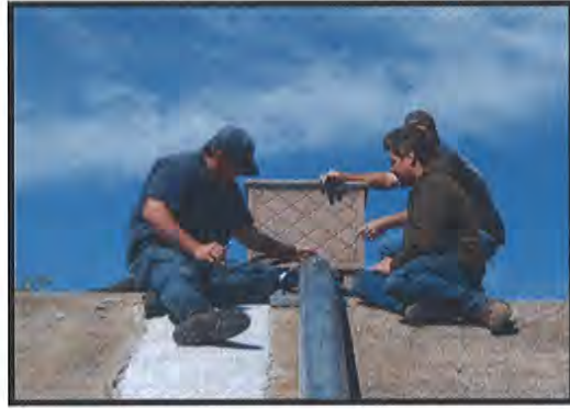
New Stafford Lake Aeration Pump
