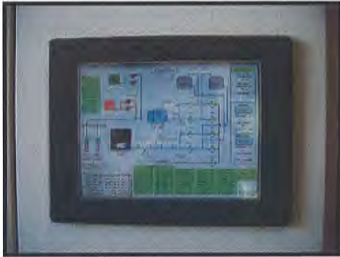
Pt. Reyes Automation Controller
