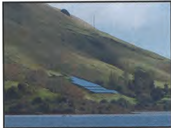
Stafford Lake Solar Power Installation
