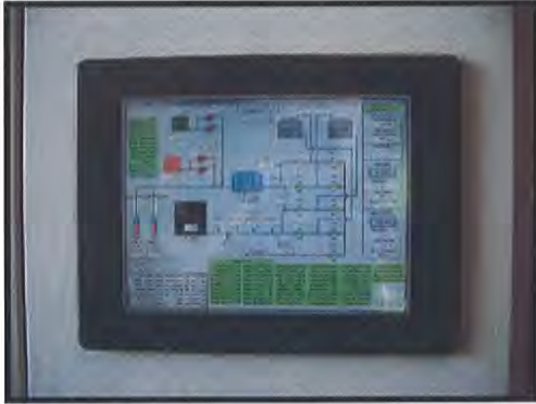
Pt. Reyes Automation Controller
