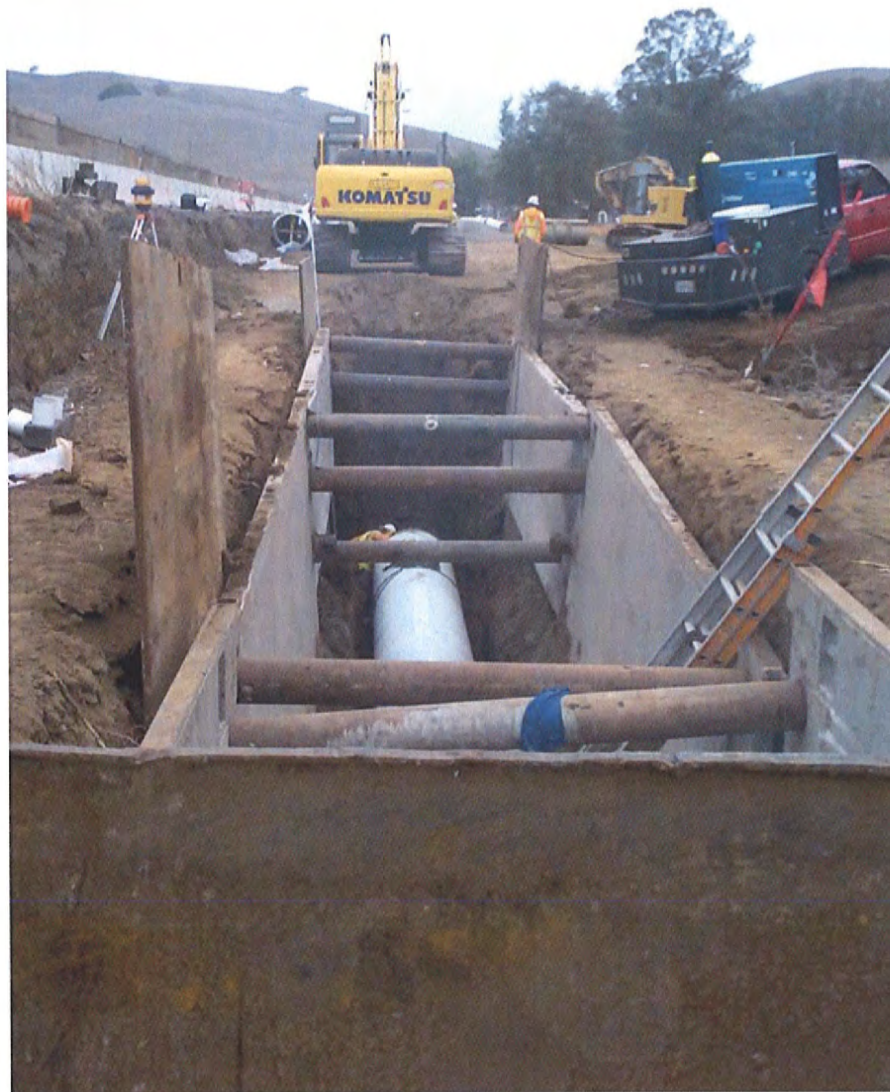
Pipe Installation Looking North from the Jacking Pit, North of San Antonio Creek
