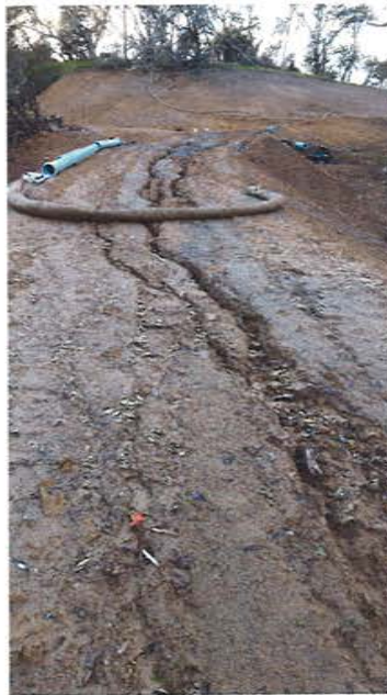
Road Erosion due to Rains
