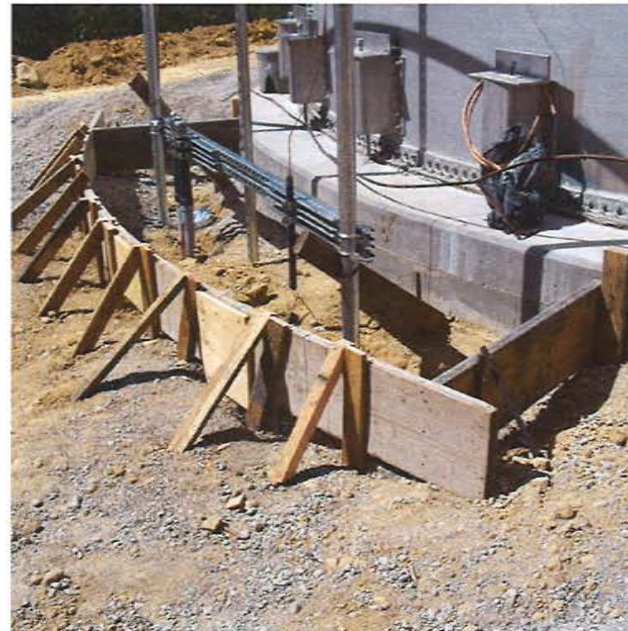
Concrete Pad for Cabinets
