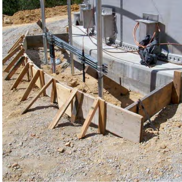
Concrete Pad for Cabinets
