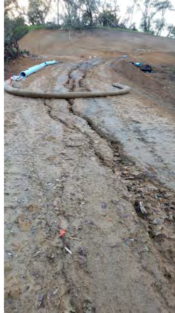
Road Erosion due to Rains
