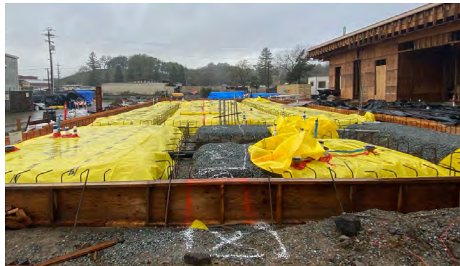
Ready for Rain
