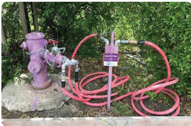
Novato residential recycled water fill station.
