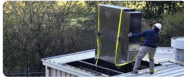
Stafford Treatment Plant High-Service Pump Station variable frequency drive replacement.
