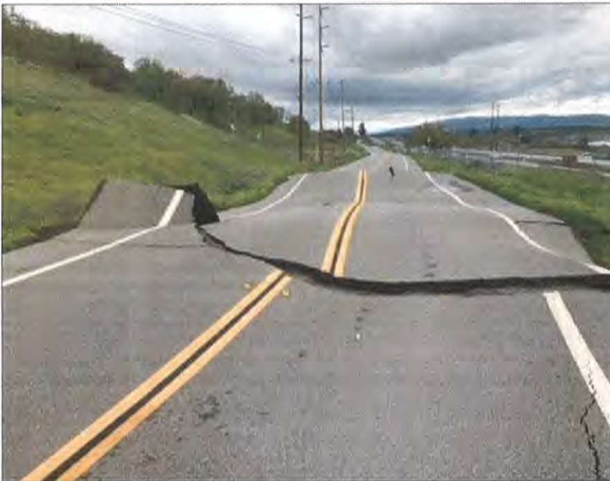
This is the scene at the Novato mudslide in the area of Olompali State Historic Park.
