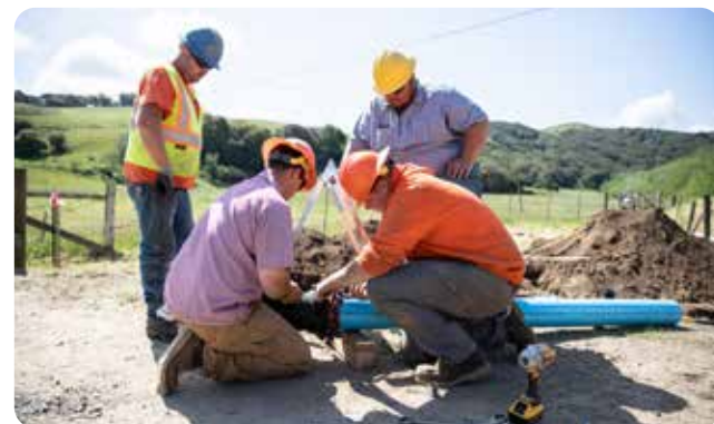
Gallagher Well No. 2 pipeline.
