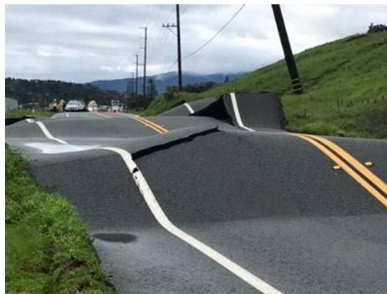
Figure 377: Mudflow damage to Redwood Blvd. March 21, 2023
