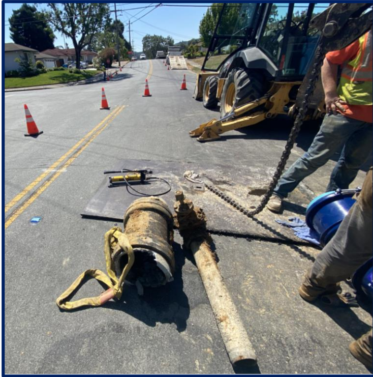
Outdated 4" Hydrant Main
