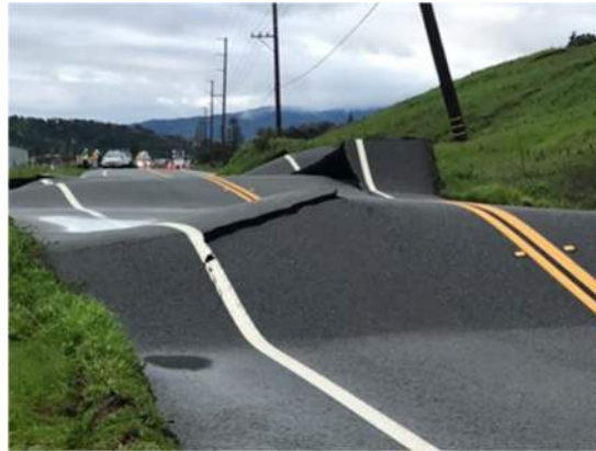
Figure 32: Mudflow damage to Redwood Blvd. March 21, 2023
