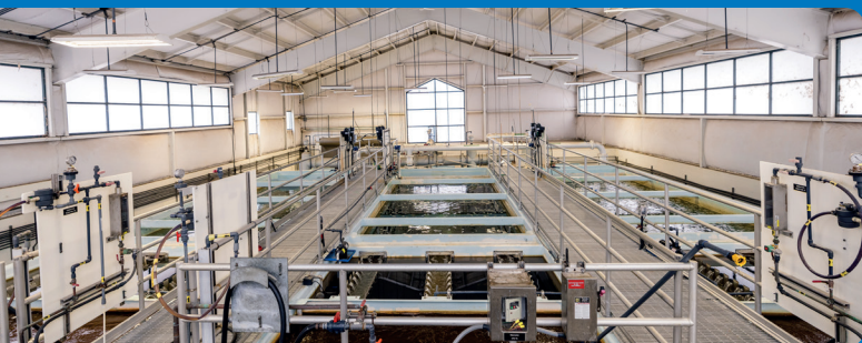
Stafford treatment plant.
