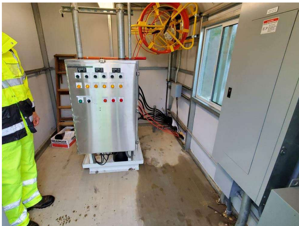
Photo 5: View of the inside of the control house on the crest at the right side of the dam.
