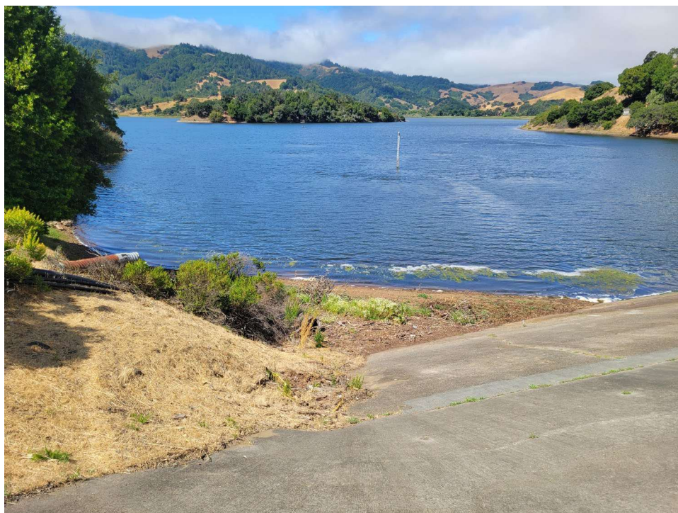
Photo 15: Photo provided by the owner on 6/25/25 of the recently removed debris from the right upstream abutment.
