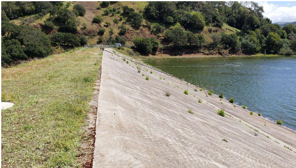
Photo 1: The condition of the crest and upstream slope liner viewed toward the right. The minor grass growth need to be removed periodically.
