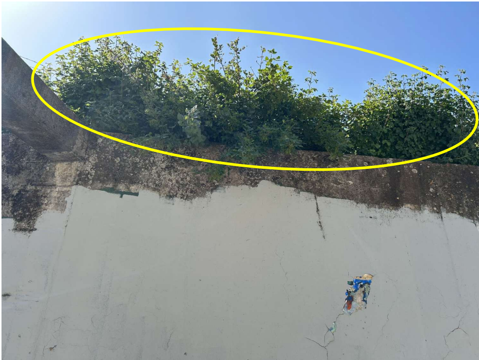
Photo 9: Remove the overhanging vegetation along the spillway channel walls (in yellow circle).
