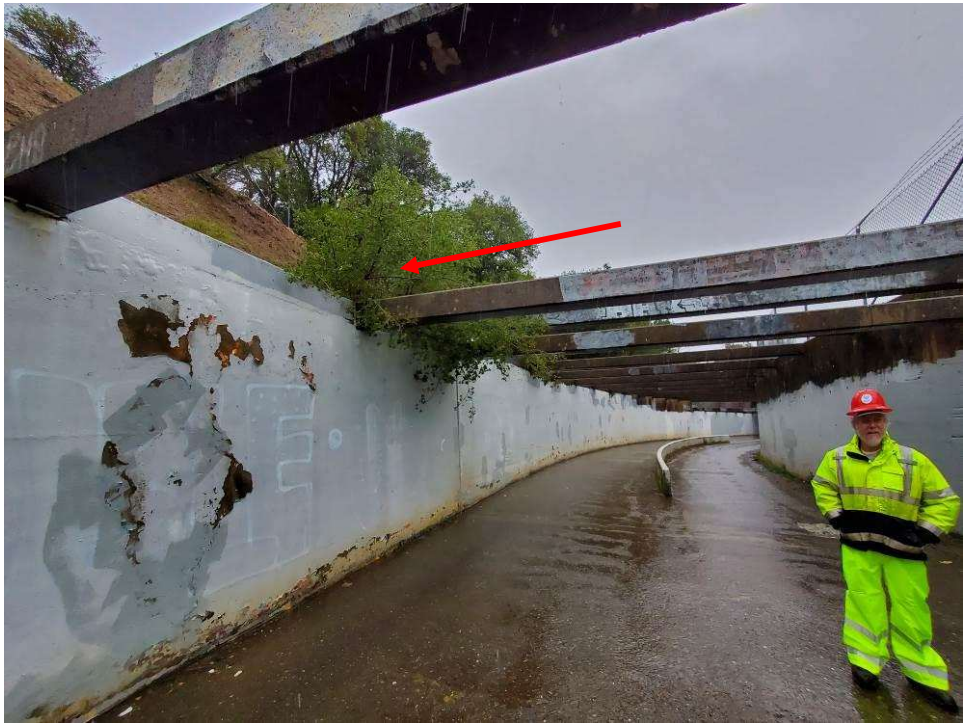
Photo 3: View of the concrete spillway chute looking downstream. The vegetation growing above the spillway wall (red arrow) needs to be removed.
