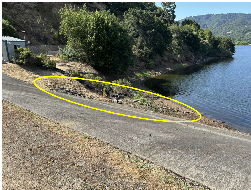
Photo 11: Remove debris from the right upstream abutment (in yellow circle).
