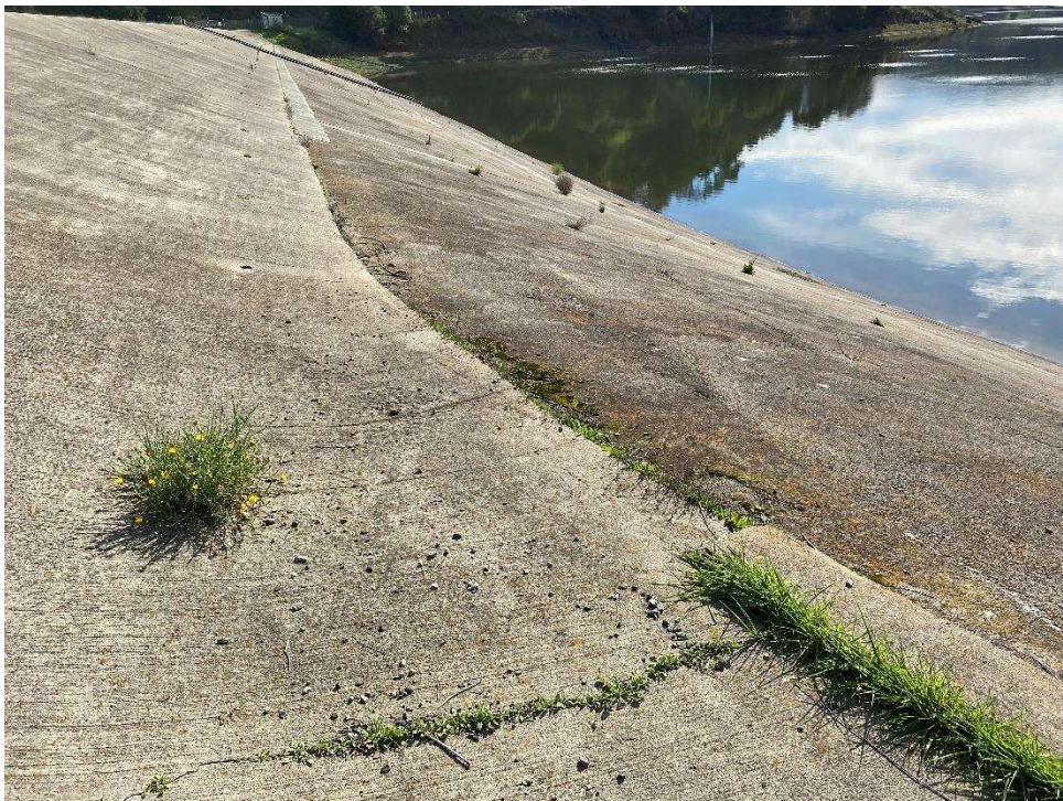
Photo 2: Debris and vegetation in weep holes needs to be removed.
