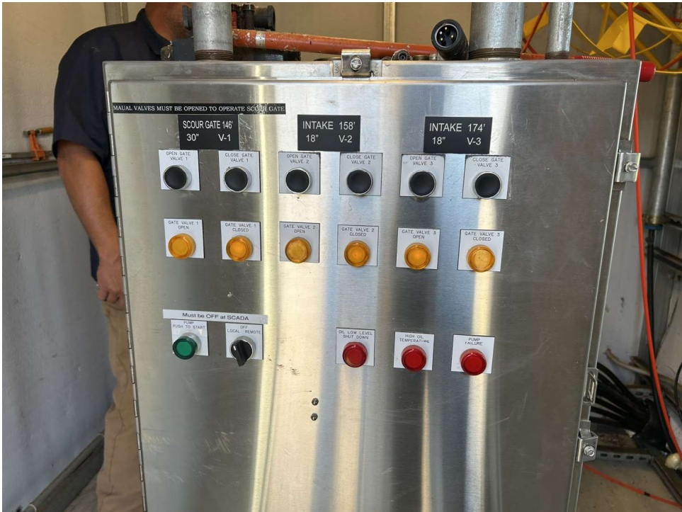
Photo 5: View of the low-level outlet controls from the control house.
