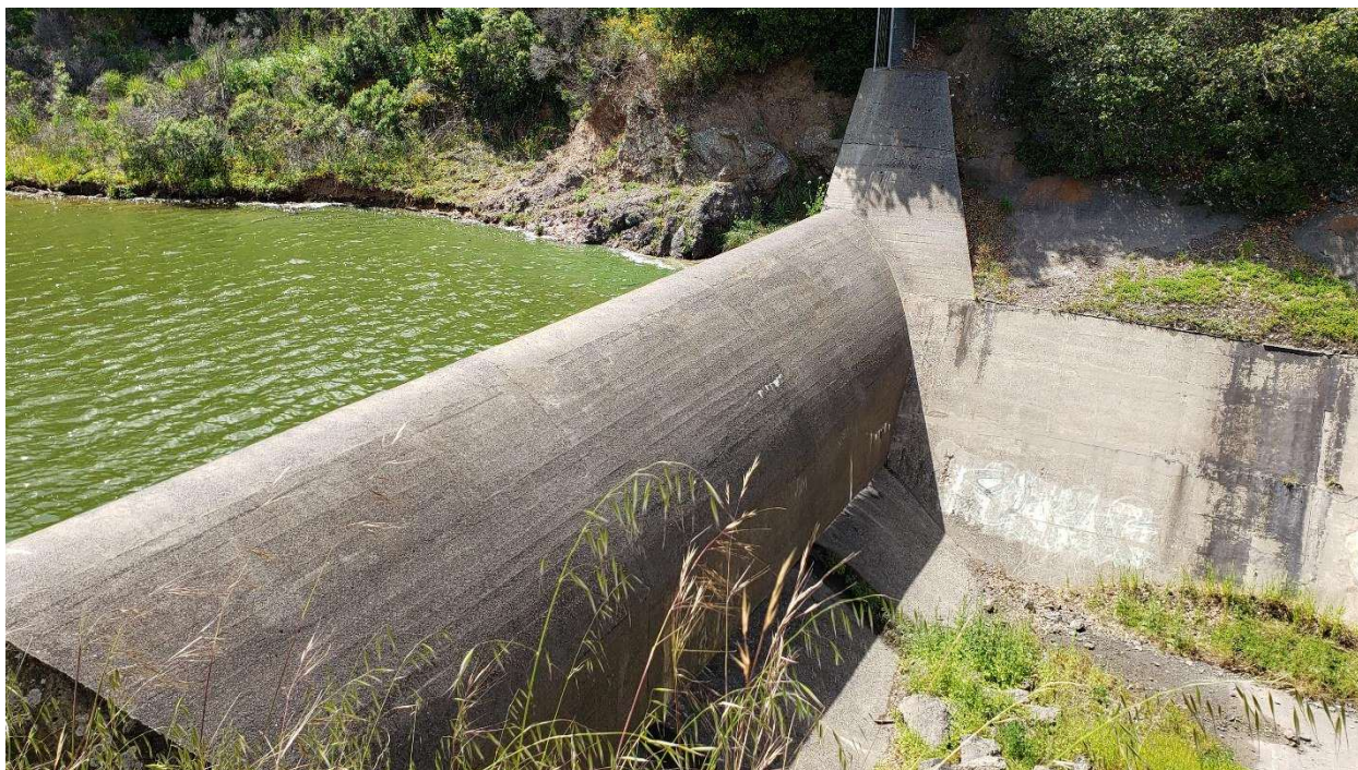
Photo 3: The ogee weir spillway control. As previously requested, vegetation growth between joints and in cracks of the spillway weir need to be routinely scraped away to prevent further damage to the concrete.
