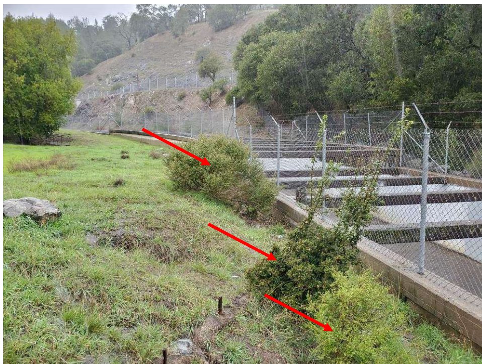
Photo 4: View of the right-side spillway chute wall. The large woody vegetation (red arrows) needs to be removed. Vegetation should be maintained at least 3 feet back from the wall.
