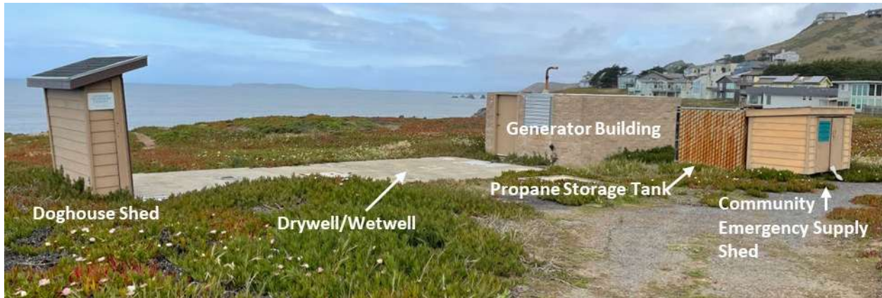
Figure 1-2. Oceana Marin Main Lift Station
