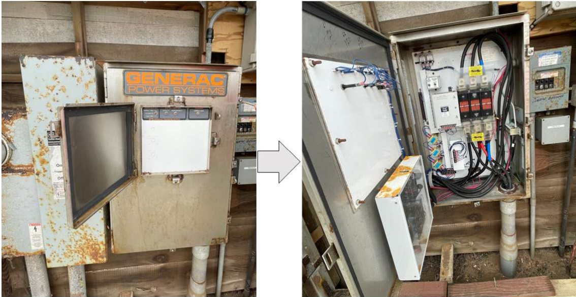
Figure 1-5. Generator Transfer Switch
