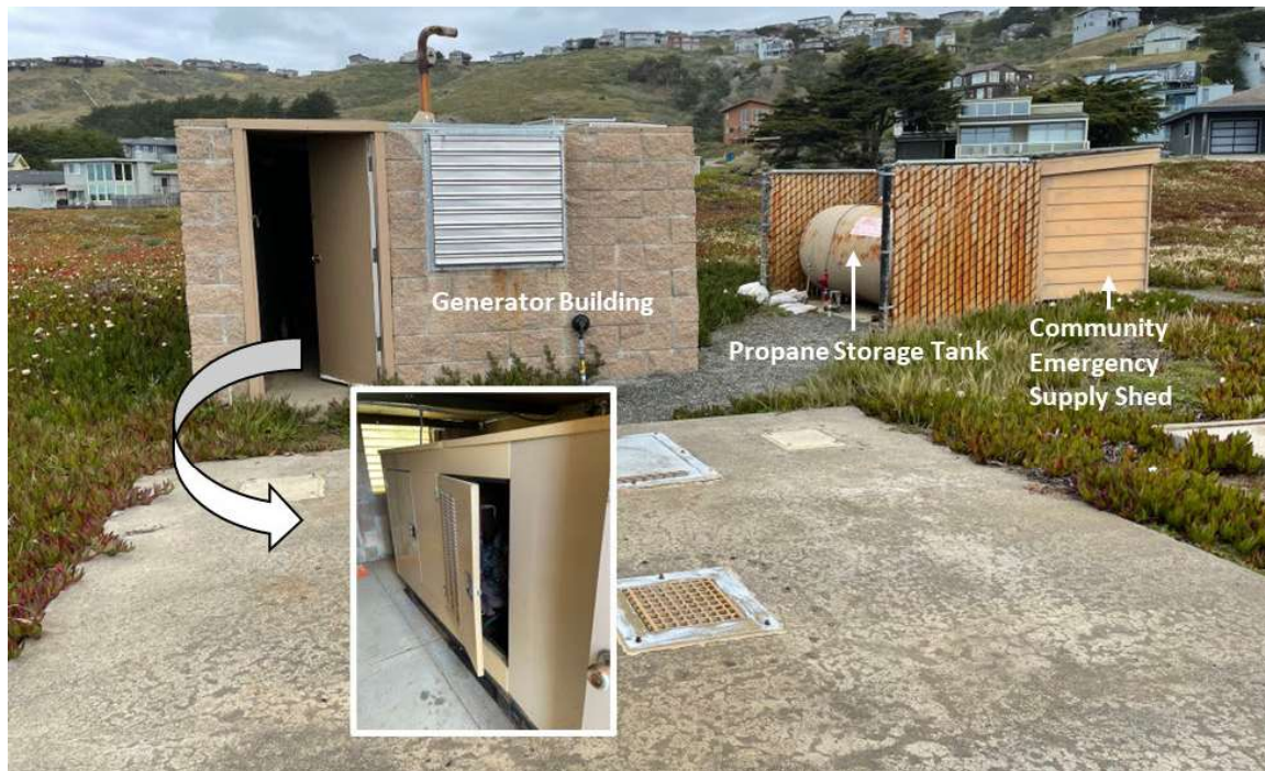
Figure 1-4. Generator Building, Fuel Tank, and Community Storage Shed
