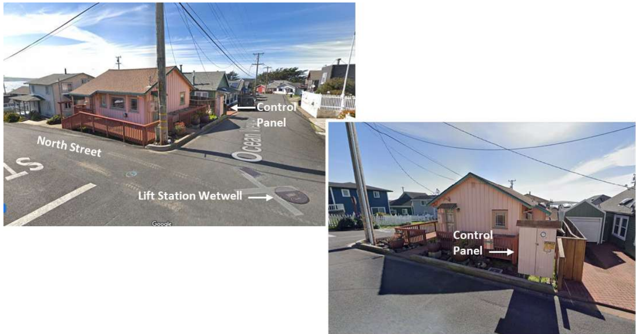
Figure 1-8. Oceana Marin North Street Lift Station
