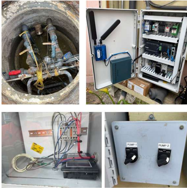
Figure 1-9. North Street Lift Station Wetwell and Electrical/Control Panel
